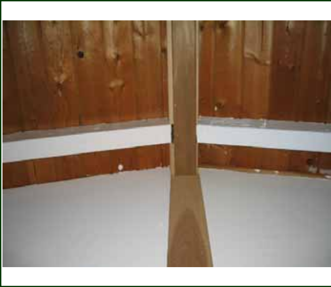
PHOTO 9: Living room rafter/ridge beam separation
