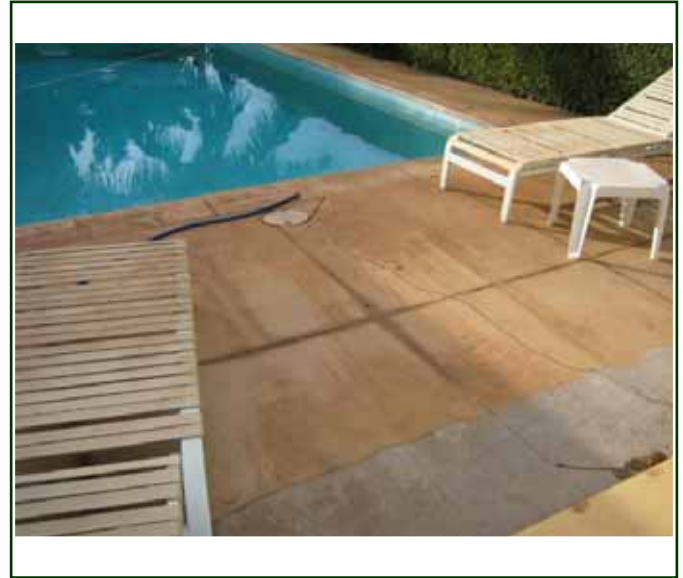
PHOTO 14: Cracks to the concrete deck at the pool
