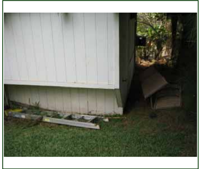
PHOTO 6: Dry rot damage to the exterior siding and a faulty grade at the left rear of the ohana
