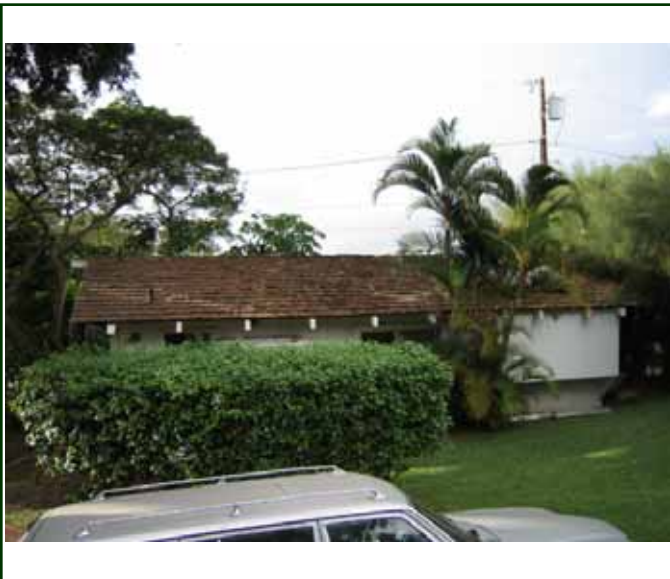
PHOTO 3: View of ohana roof, note debris on the right side and trees in contact with the roof
