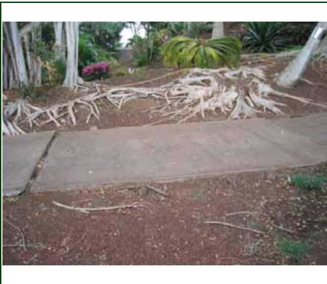
PHOTO 11: Root damage at the driveway
