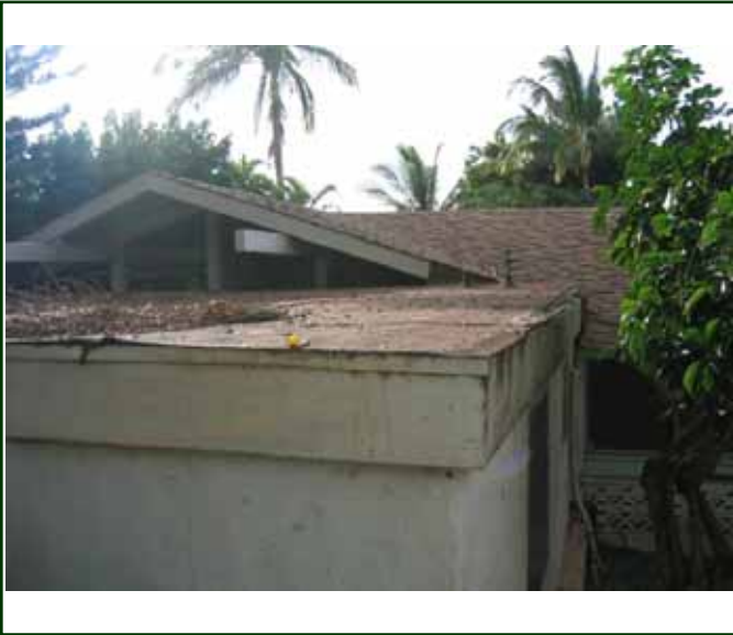
PHOTO 13: Flat roof section over the main house addition. Note damage to wood fascia board at the side and rear
