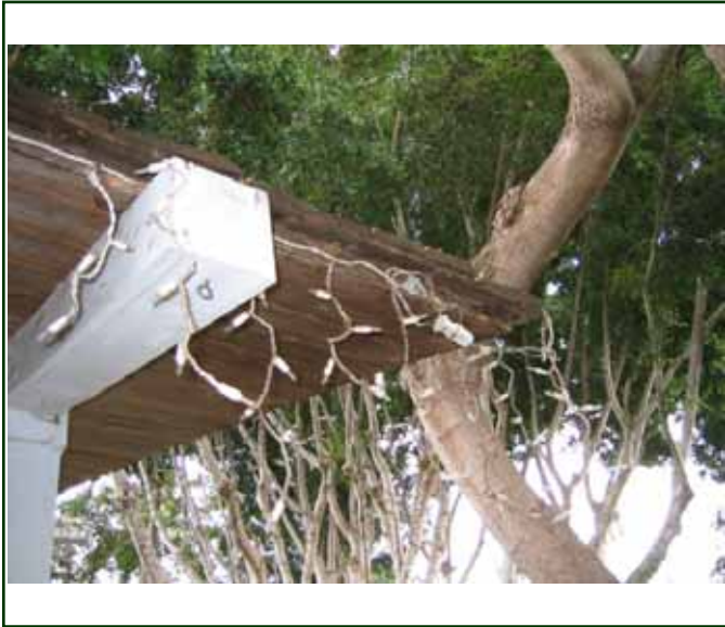
PHOTO 5: Insect and possible water damage to the eave at the left front corner of the ohana
