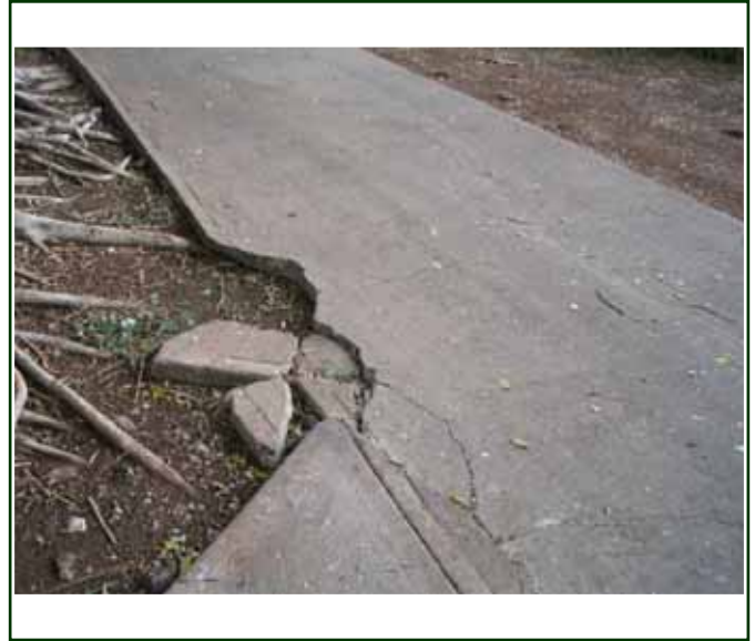
PHOTO 10: Root damage at the driveway
