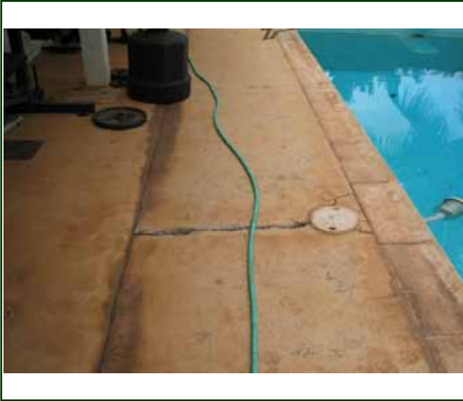
PHOTO 1: Cracks and separation at the pool decking
