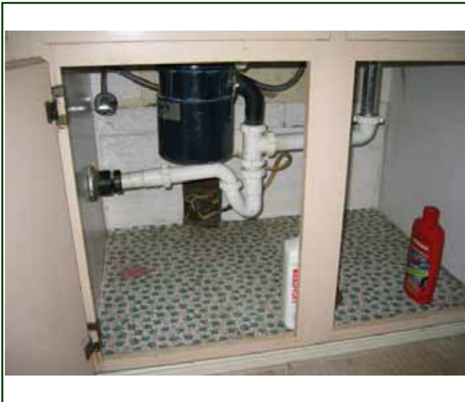
PHOTO 7: Exposed electrical splice at the disposal under the ohana kitchen sink
