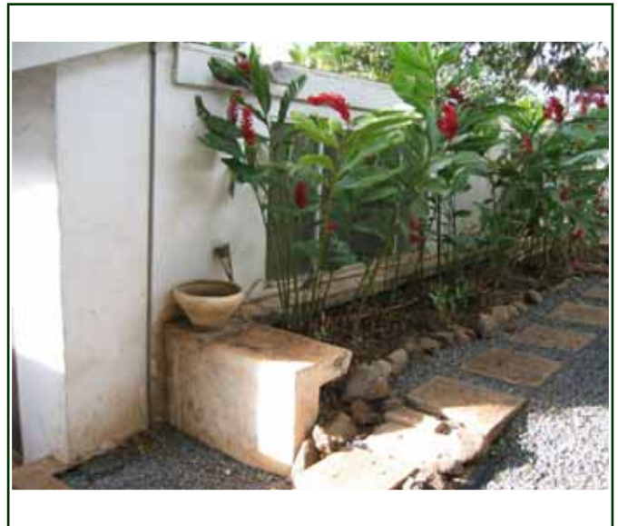
PHOTO 12: Faulty grade at the main house addition
